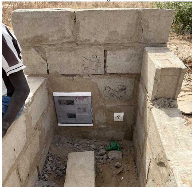
Electric meter installed on a vegetable farm in Bâko Dior
